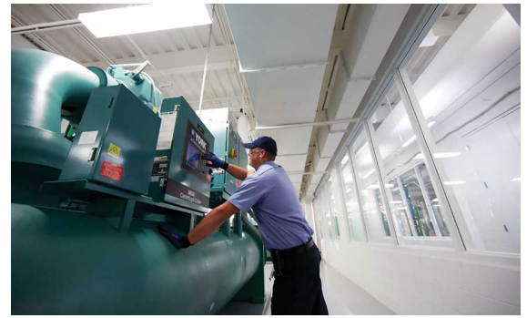
OPTIMIZED EQUIPMENT: Artificial intelligence may allow companies to optimize not only equipment such as chillers, but also their operations. PHOTO COURTESY OF JOHNSON CONTROLS INC.
